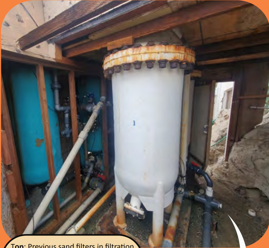
Top: Previous sand filters in filtration room at KML.
